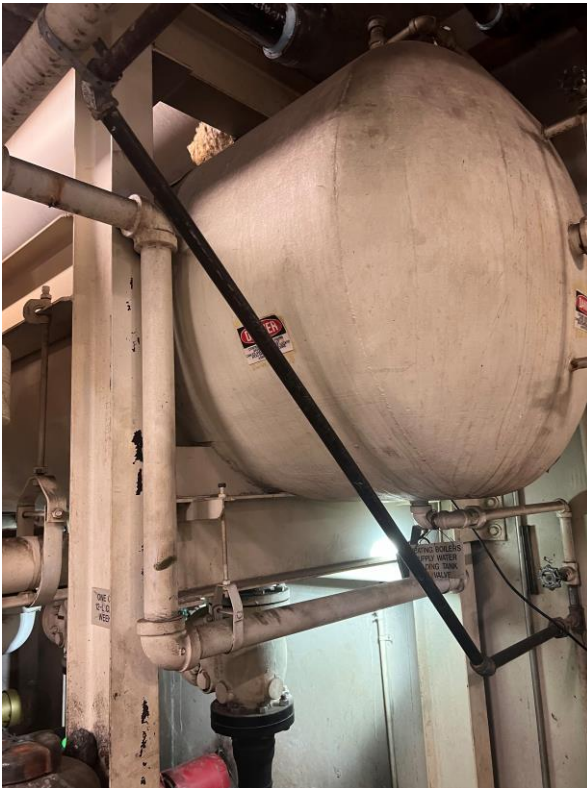
Picture 18: Expansion Tank 3
