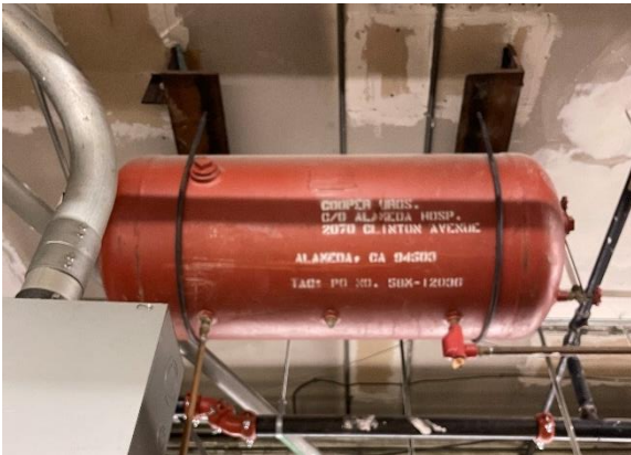
Picture 11: Expansion Tank 1
