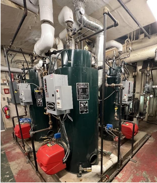
Picture 19: Existing Central Steam Generators
