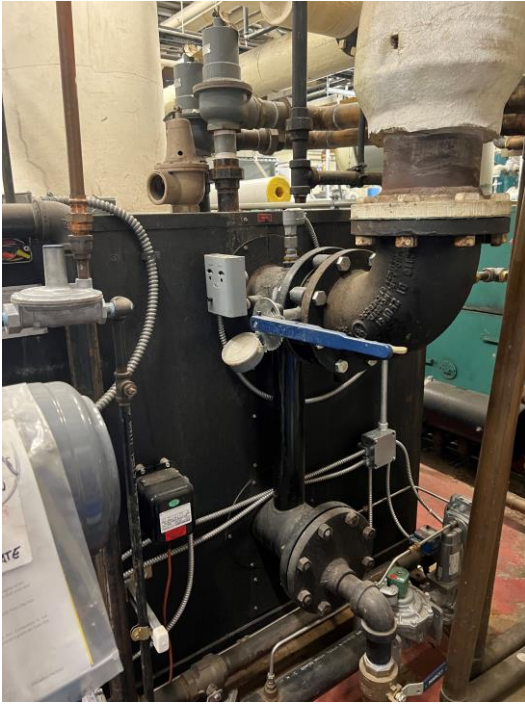
Picture 12: Existing Boiler #1
