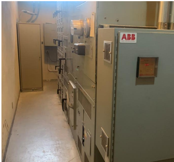
Picture 19: Existing main Switchgear 'MSB'.
