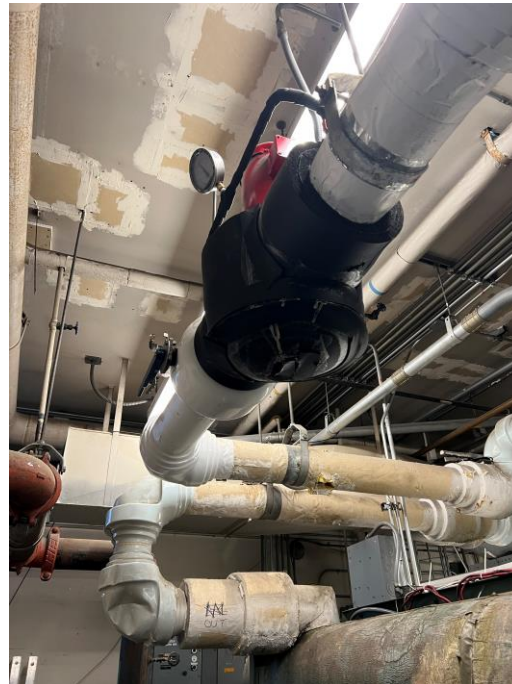
Picture 6: Chiller #2 Primary Chilled Water Pump (P-9)
