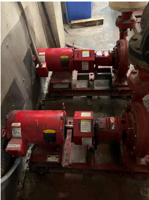
Picture 16: South Wing HHW Pumps P-3 and P-4
