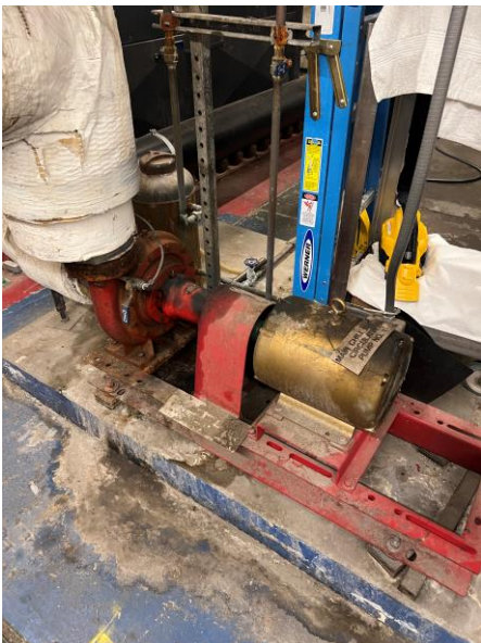
Picture 9: South Wing Chilled Water Pump (P-1)
