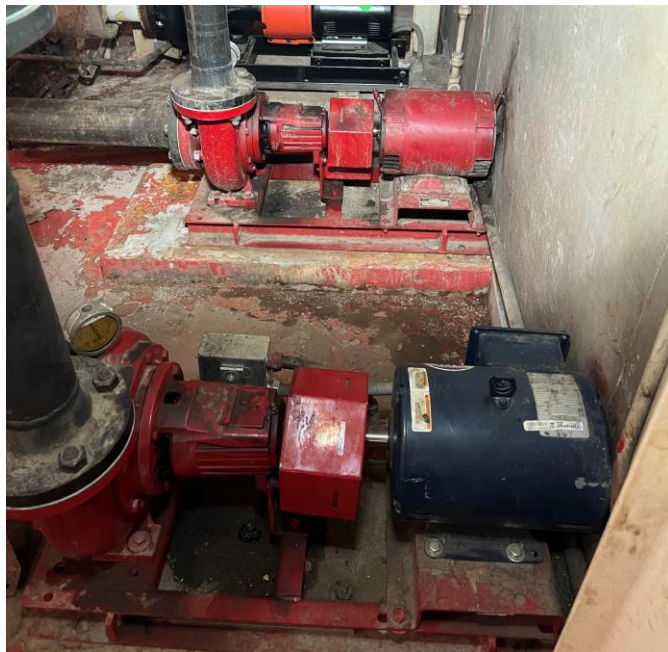
Picture 17: West Wing HHW Pumps P-10 and P-11
