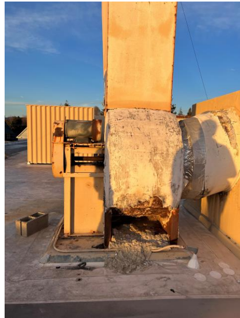
Picture 15: Gas Flue Exhaust Fan
