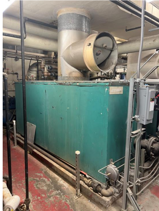
Picture 13: Existing Boiler #2
