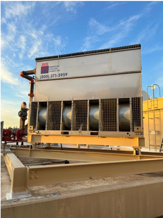
Picture 3: Existing Cooling Tower #1
