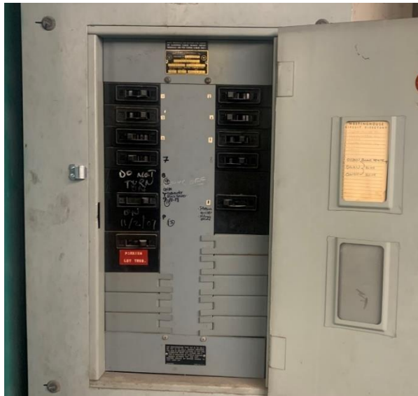
Picture 20: Existing panel 'BE'.
