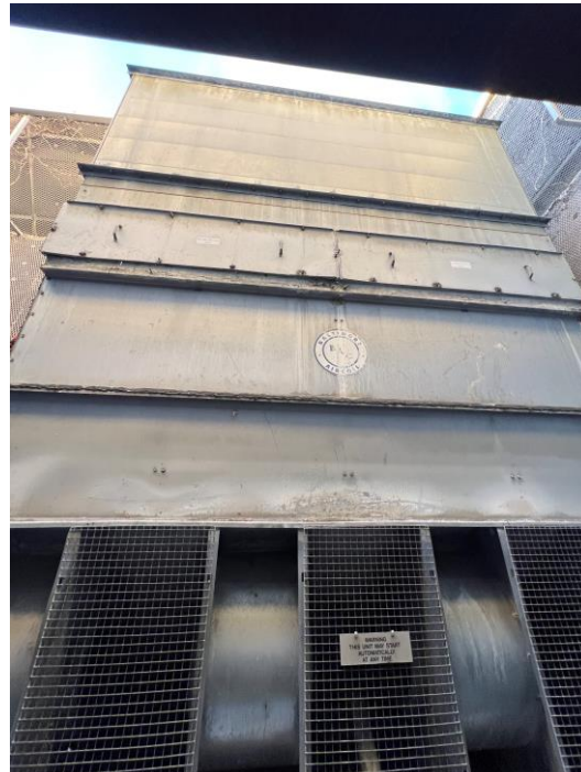
Picture 4: Existing Cooling Tower #2
