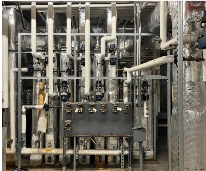
Picture 20: Existing Steam Humidifiers
