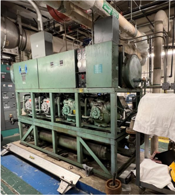
Picture 1: Existing Chiller #1
