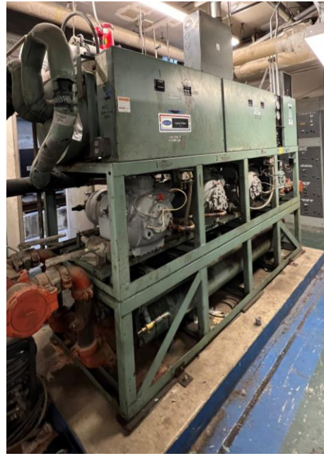
Picture 2: Existing Chiller #2
