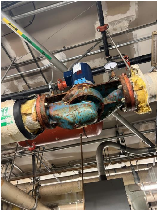
Picture 5: Chiller #1 Primary Chilled Water Pump (P-8)
