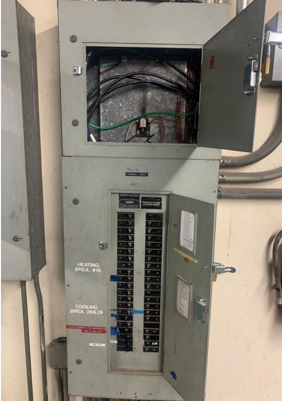
Picture 21: Existing panel 'BET'.
