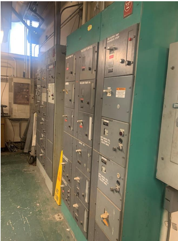
Picture 23: Existing motor control center 'MCC-2'.
