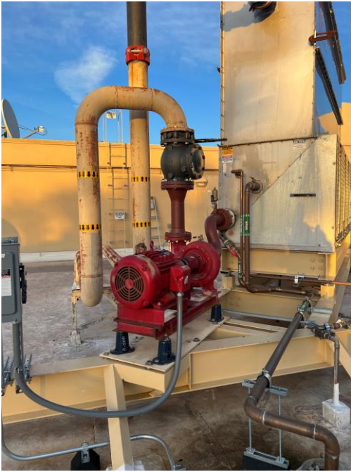
Picture 7: Chiller #1 Condenser Water Pump (P-2)
