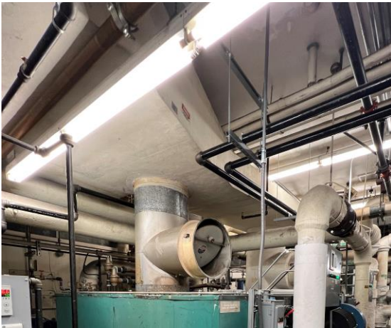
Picture 14: Gas Flue Exhaust
