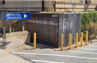
EXISTING FUEL STORAGE TANK
